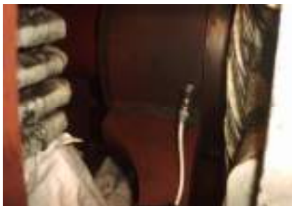
Fig. 7 The 8 th bearing SPM2 transducer installed on the bearing housing inside generatortion
