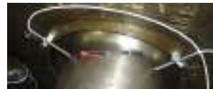
GR 7 th bearing shaft with installed two contact less vibration displacement measurement sensors 7Y (left) and 7X (right)
